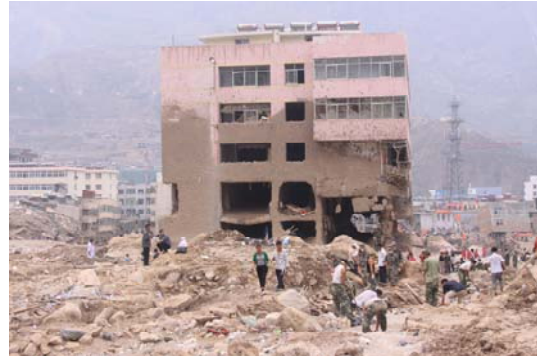
The building was damaged
