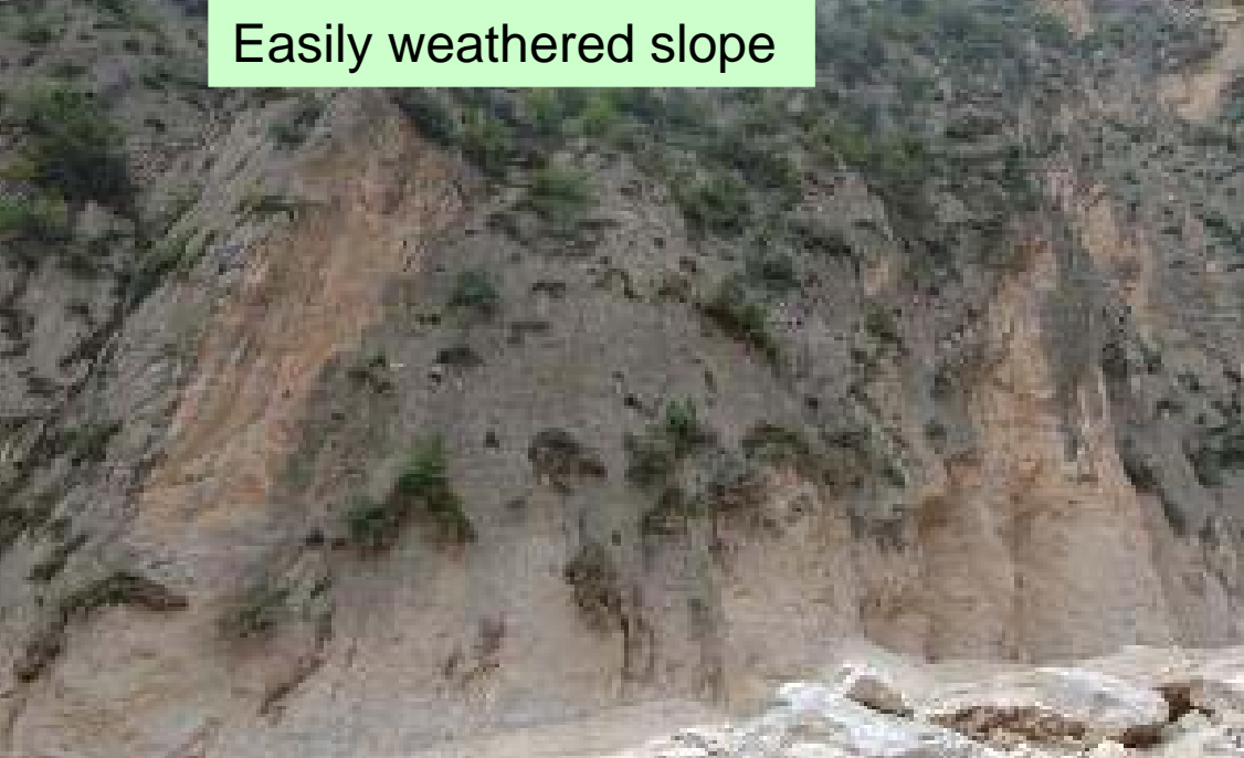
Unsteady loose materials
